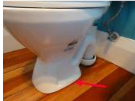
Sealant would be beneficial.
