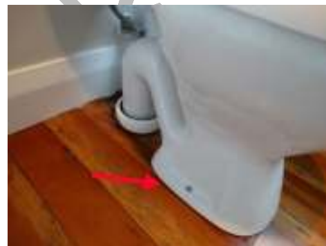
Sealant would be beneficial.
