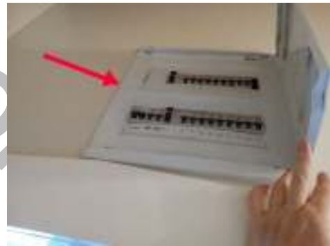
Door fell off when opened.
