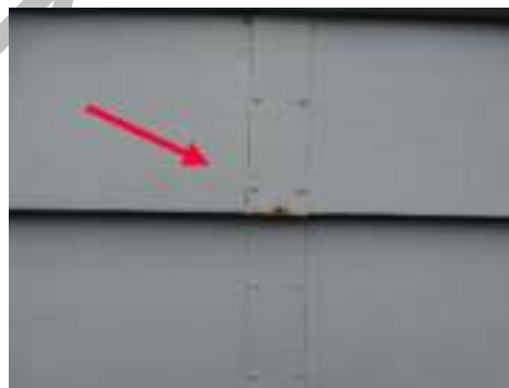
Minor corrosion noted.
