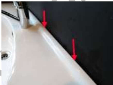
Sealant would be beneficial.
